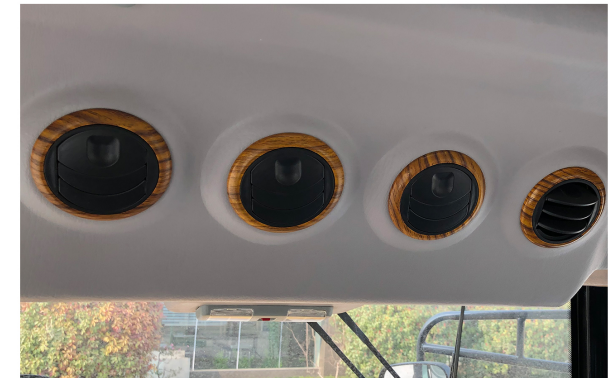
Heating and cooling air conditioning
